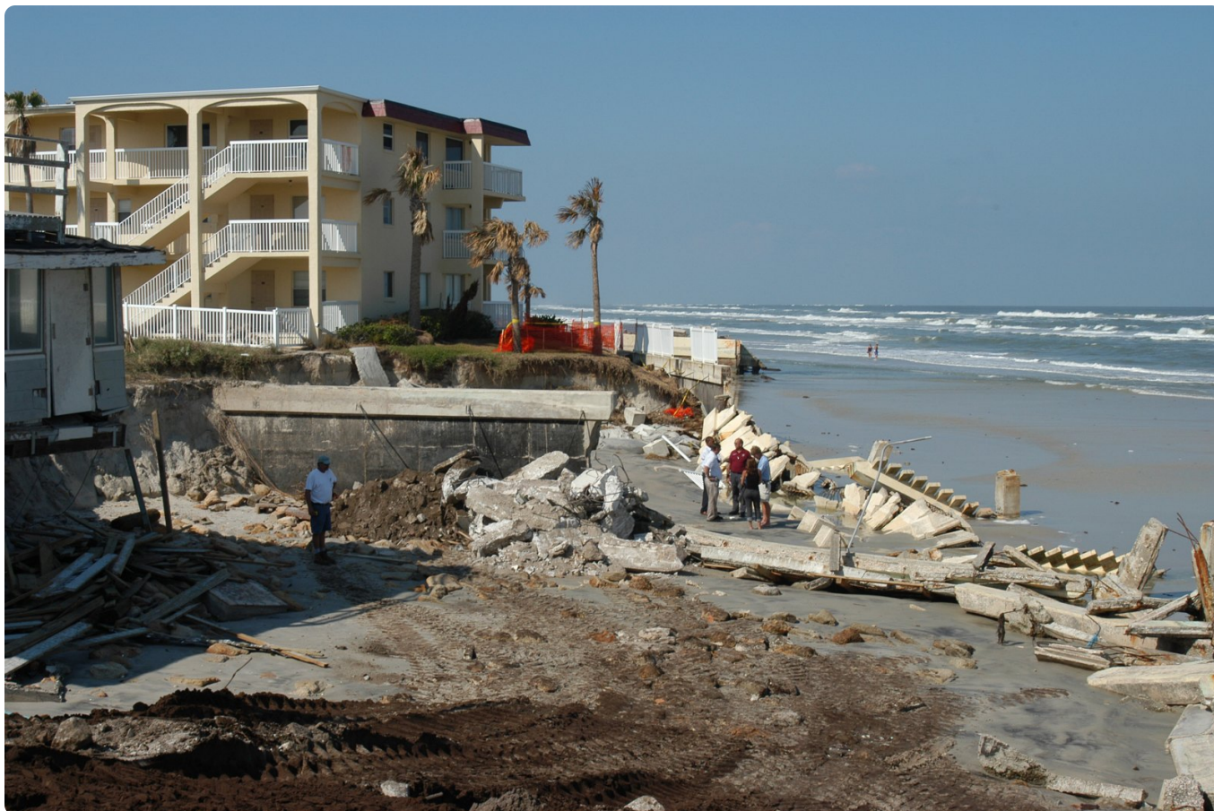
A seawall left standing with the fill washed out behind it. New Smyrna Beach, Florida, October 2004. Photo: FEMA / Mark Wolfe.
